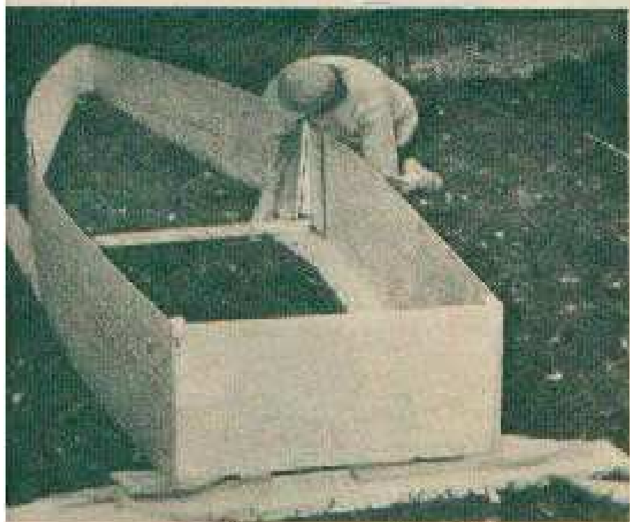
FASTEN SIDES to stem, mid-frame, transom. Spot mid-frame \frac{1}{2} in. ahead of butt joint.
